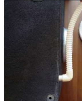
Inserting the line and securing it with a clip (the clip and the line is provided by the plumbing installation company)
